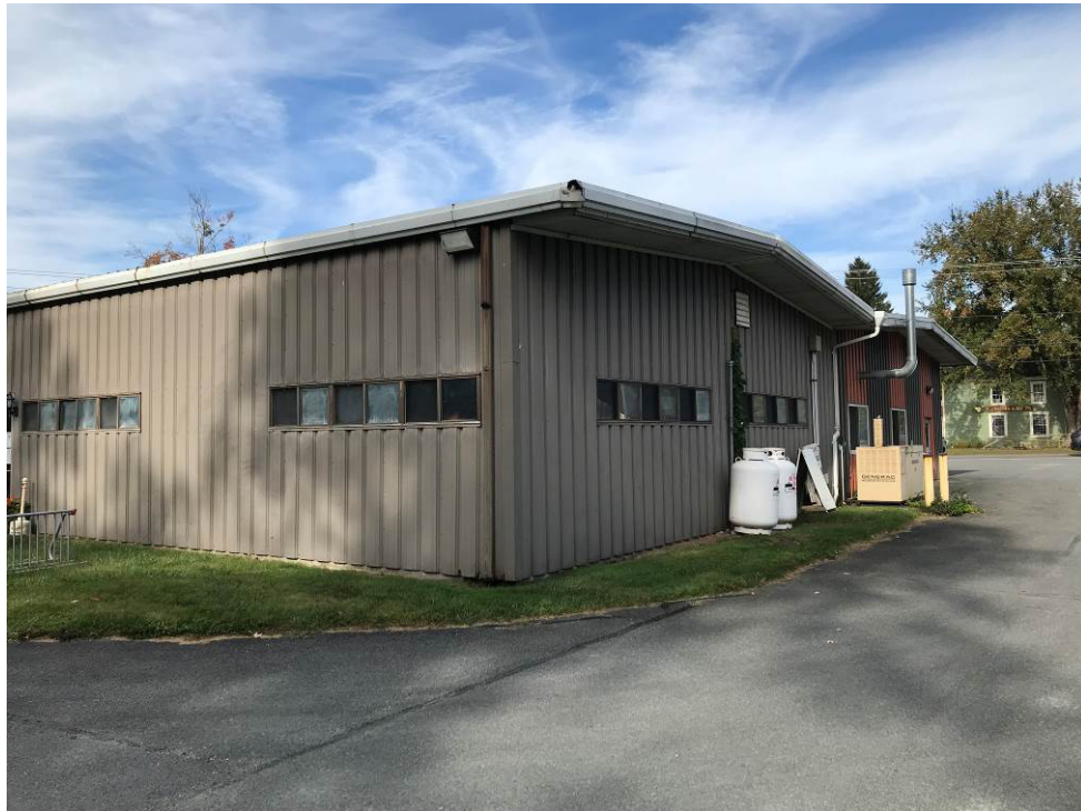
Window Caulk at Brown Windows
