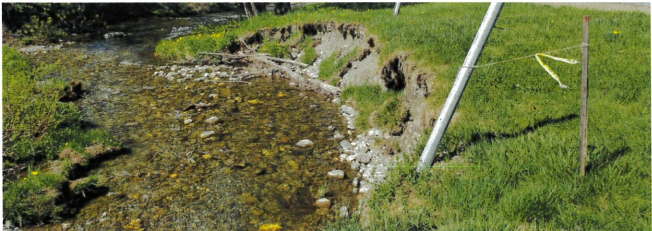
POWERS, S. 2024. SHATFORD PARK CREEK EROSION NEW LEBANON, NY
