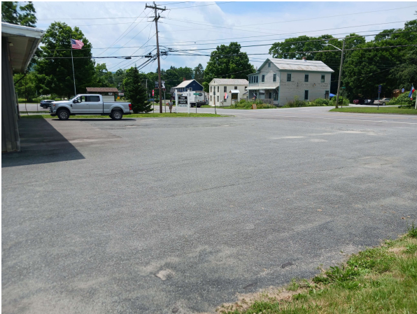
Photo 5: Front Parking Area
