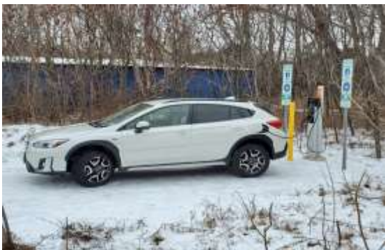
A resident uses New Lebanon's new EV charging station
