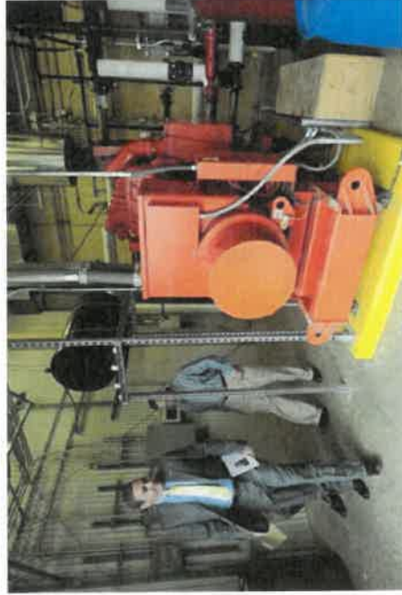
City of Schenectady CHP Project
